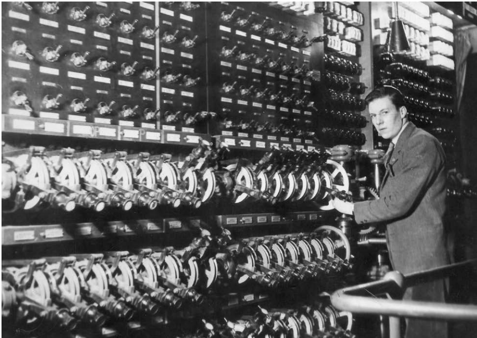
Figure 6. Electric Strand’s Grand Master lighting control. Photograph courtesy of Andy Collier.
